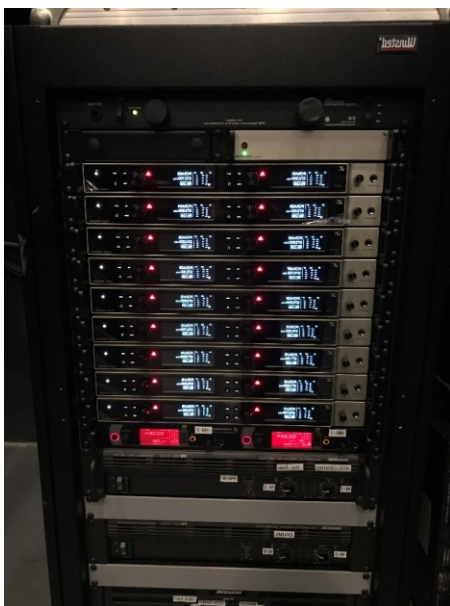
One of the Sennheiser racks at WKAQ
